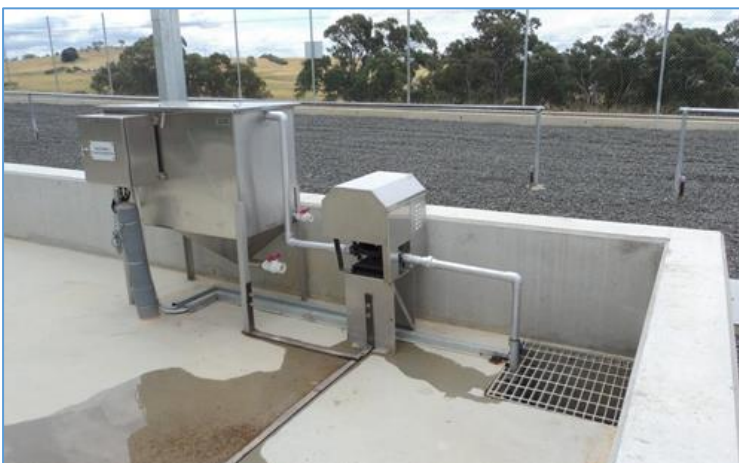
Figure 7: Oil / water separator within bund of Transformer 2.
