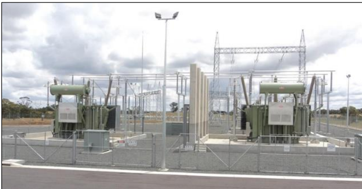
Figure 6: 33kV / 330kV substation including the two banded transformers.
