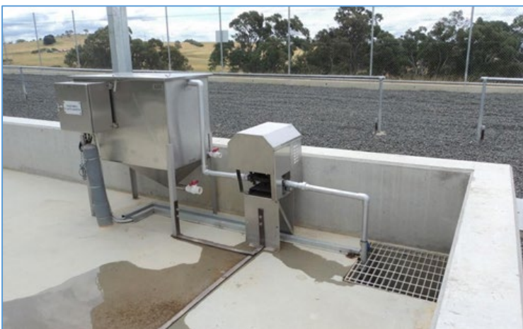
Figure 7: Oil / water separator within bund of Transformer 2.
