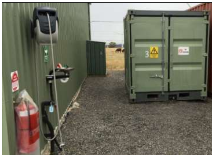
Figure 4: Onsite chemical storage container at Site O&M Compound.
