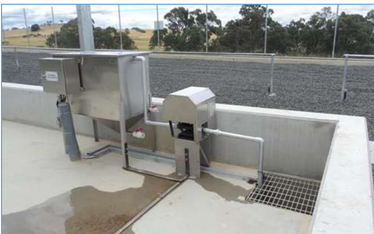
Figure 7: Oil / water separator within bund of Transformer 2.
