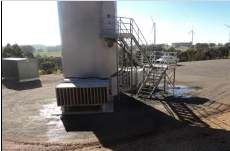
Figure 2: Lower portion of a GW100 2.5MW turbine.
